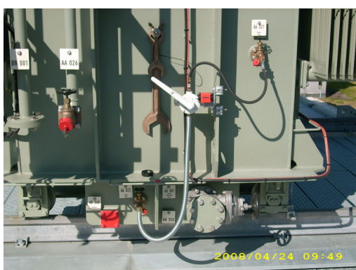
Fig. 1 Oil Pump Installation (OPI)
